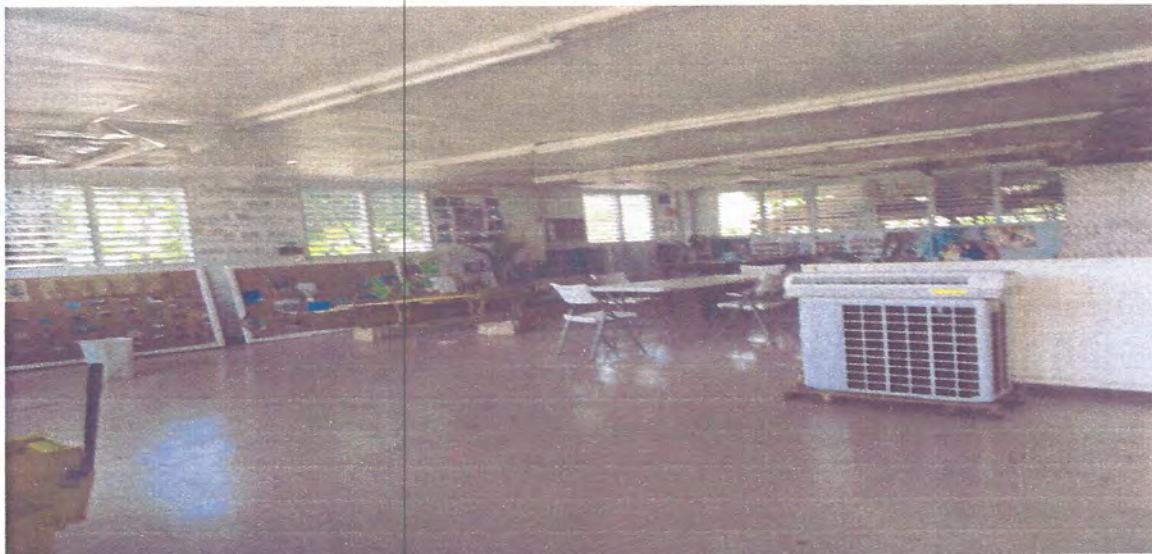
70 Pohnpei Visitors Bureau - Ceiling almost fall apart.
