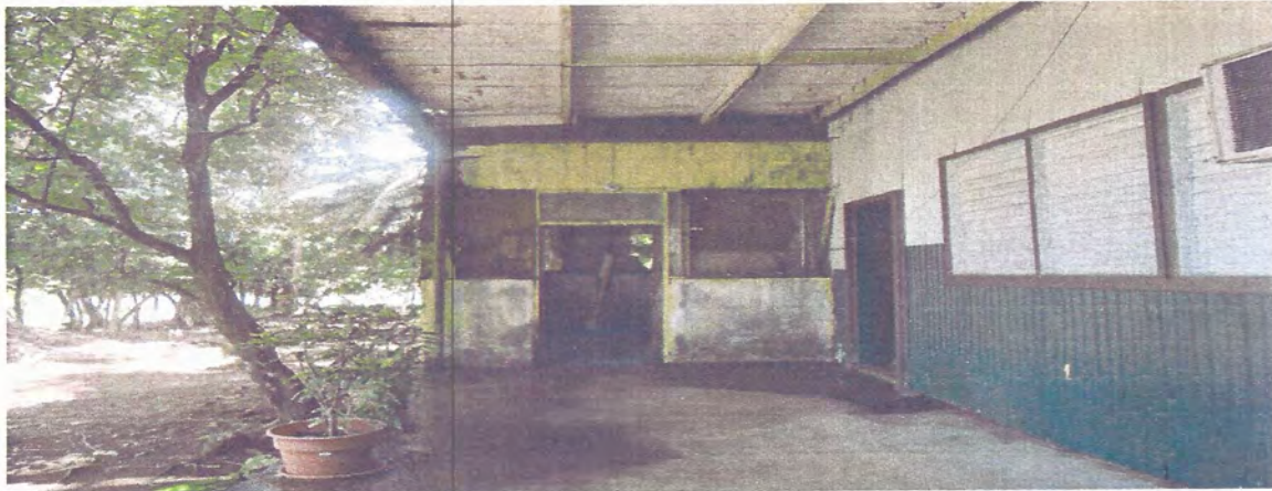
58 Pohnpei Visitors Bureau -Entrance area is dilapidated
