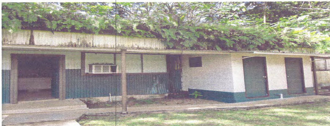
71 Pohnpei Visitors Bureaus - weeds grows wildly on top of the office building
