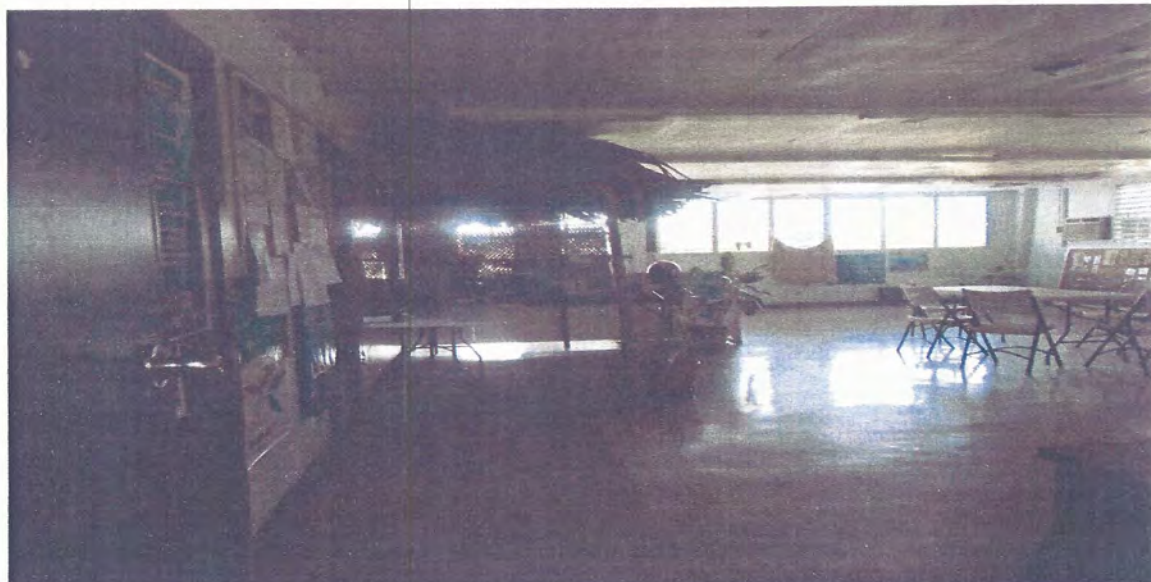
59 Pohnpei Visitors Bureau- Receiving Area- Ceiling almost collapse
