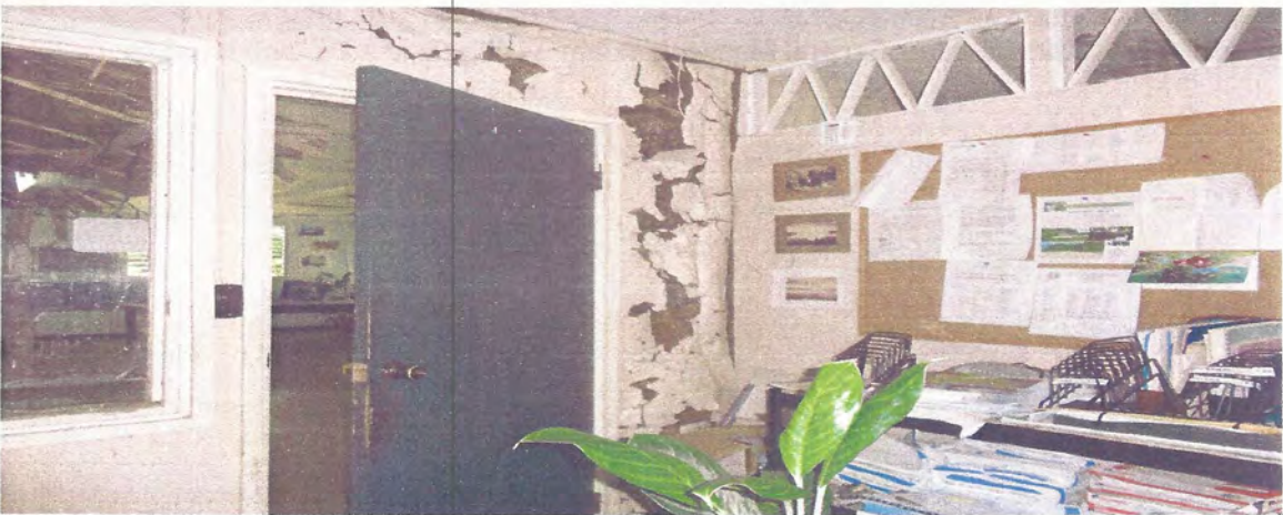
62 Pohnpei Visitors Bureau Computer Room – Ceiling and wall with termites
